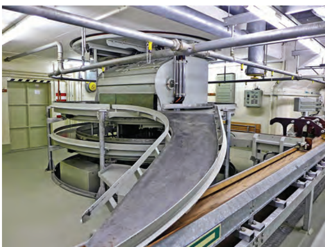
Fort Dailly: The ammunition carousel at the foot of the vertical shaft to the turret
